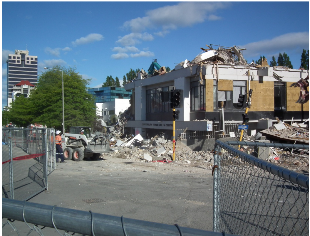
Photo above shows the TUC Building in the process of being demolished (Photo—Amanda Stephens)
